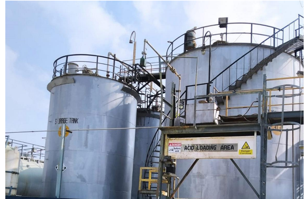
Sulfuric acid containment tanks, Qatar Acids Company (image courtesy of Qatar Acids)
